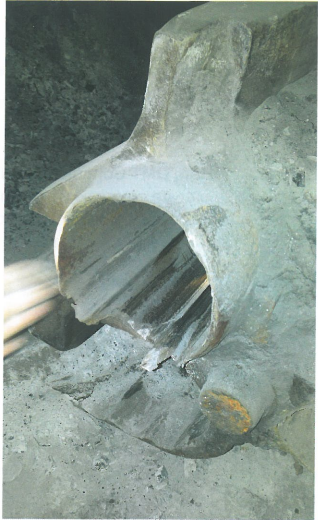
Figure 4. Damaged guide duct.
